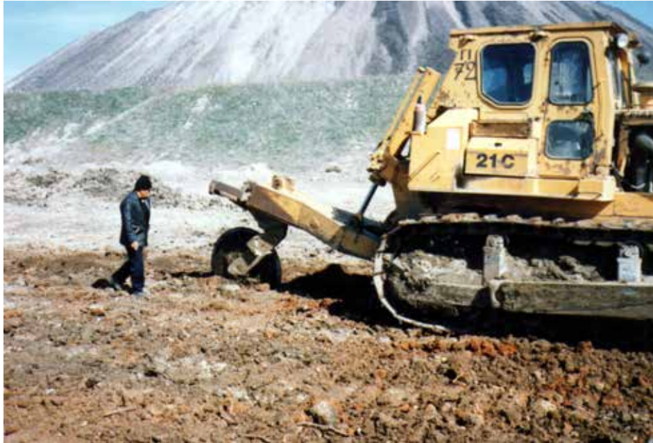
Figure 7. Spreading of topsoil with caterpillar used to cut the Robinia roots into smaller pieces
